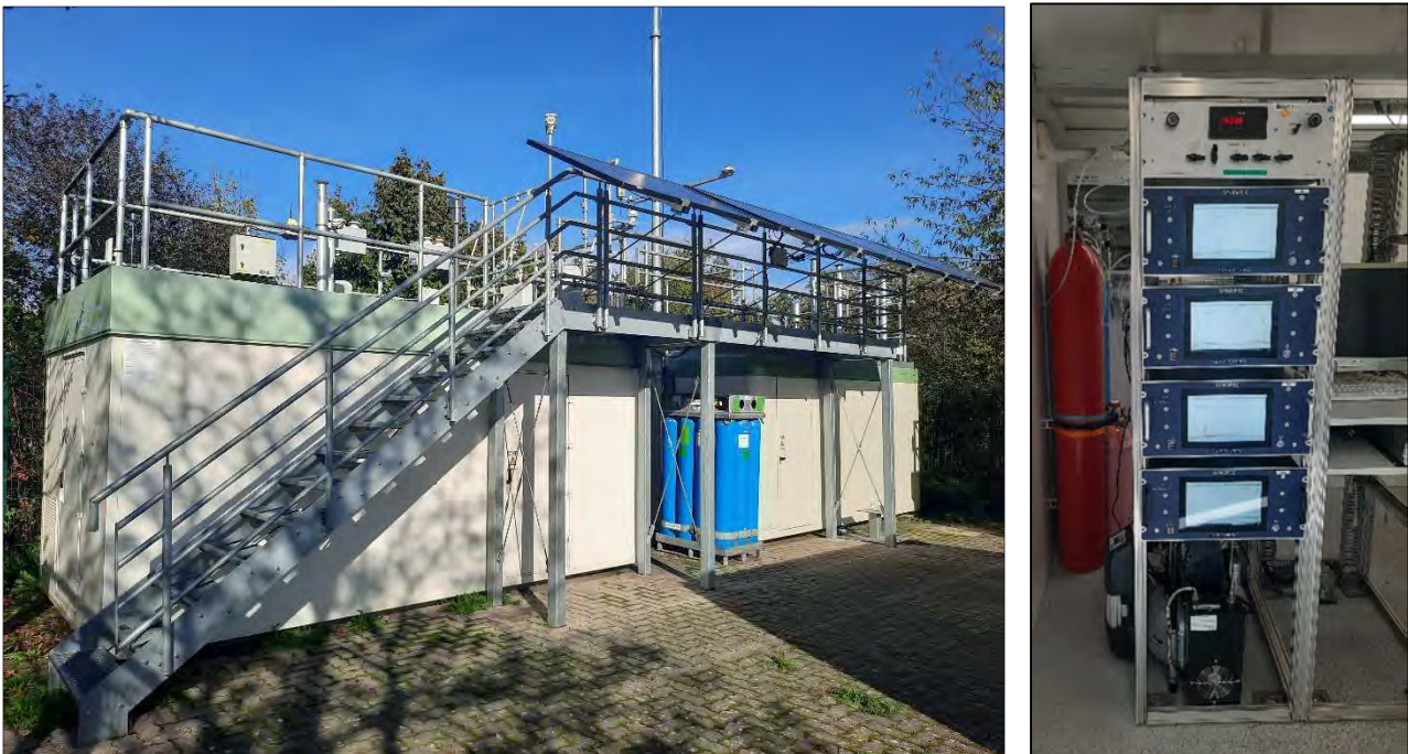
Fig. 4.1: Measuring station at the LUBW test site
