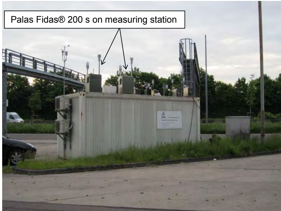
Figure 14: Fidas® 200 S measuring systems on measuring station
