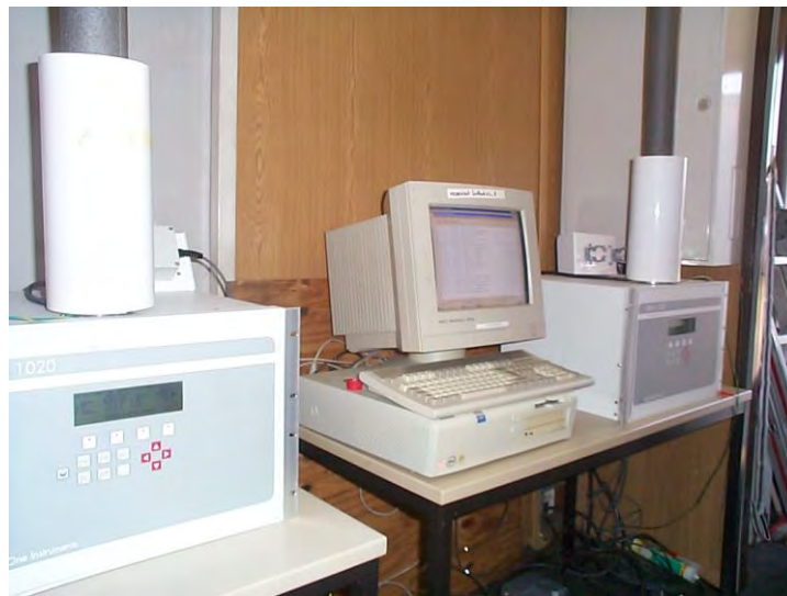
Figure 7: Measuring systems BAM-1020, installed in measurement cabinet
