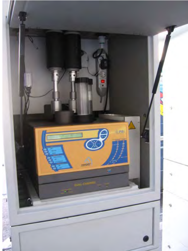
Figure 9: SWAM 5a Dual Channel Monitor installed to the outdoor measuring cabinet
