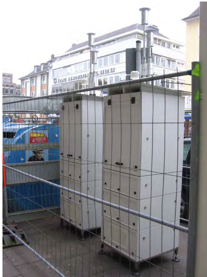
Figure 8: Outdoor measuring cabinets at the field test site in Bonn-Belderberg
