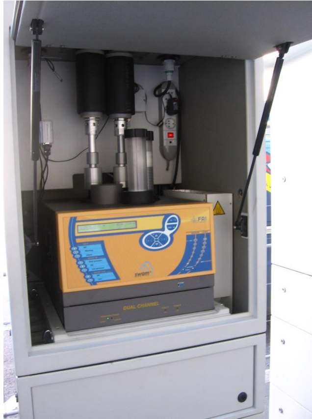
Abbildung 12: SWAM 5a Dual Channel Monitor in Outdoor-Messschrank
