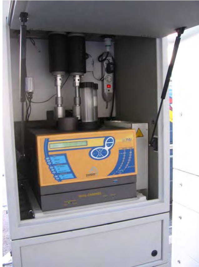
Abbildung 9: SWAM 5a Dual Channel Monitor in Outdoor-Messschrank
